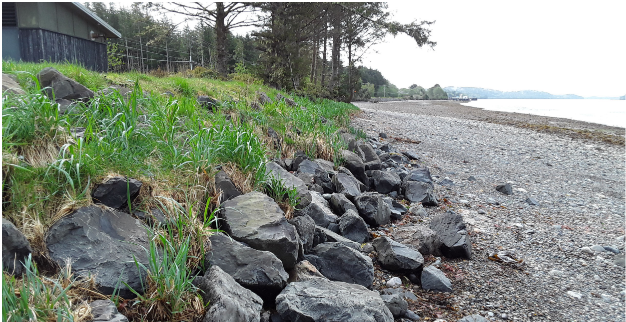
Figure 3-5. Typical west-facing shoreline in Masset Sound. Gravel and cobble material dominate the foreshore and rock armouring has been installed to address wave cutting erosion at the upper shoreline. The armour rock shown in this photo is relatively new but already showing signs of failure from undercutting.
