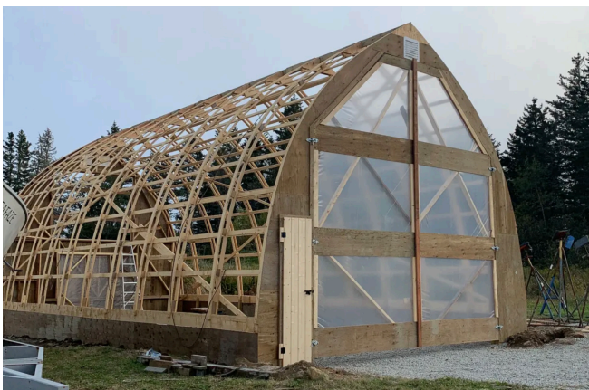
Fig 1.4 example of a bow-roof shed frame. This one is considerably taller than the one proposed.
