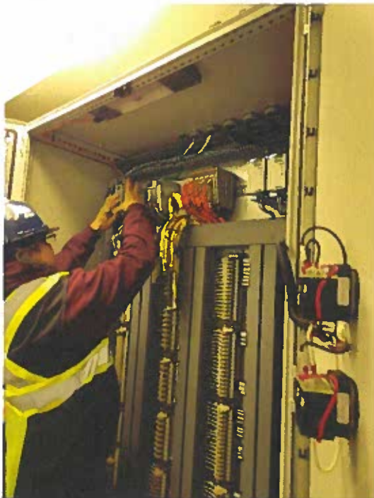
Wiring in the new PLC
