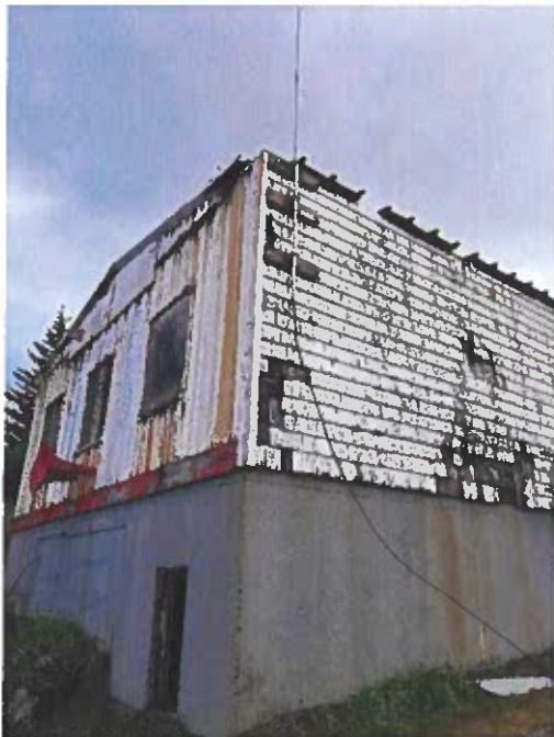
Figure 3: Siding and Foundation Cracks
